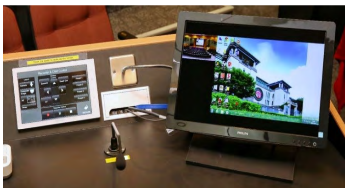
Control Panel Setup
